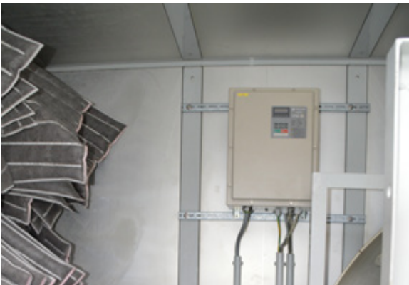
The new drive is much smaller and lighter than the old one. The compact frequency converter was mounted on the wall.
