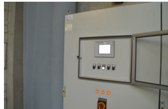
The ventilation system is still controlled manually via a potentiometer. On the left is one of the filter bellows, through which the clean air flows into the hall.
