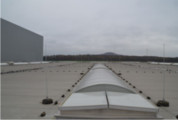
The roof area demonstrates the impressive dimensions of the bottling plant. The surrounding area is mainly forests that provide the best water quality
